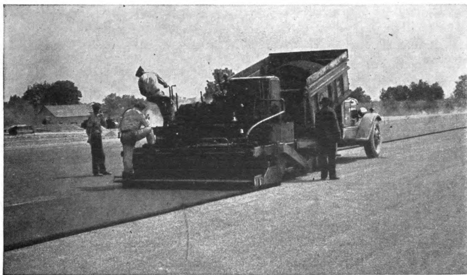
Figure 116. Spreading-and-finishing machine laying bituminous pavement. Mixture prepared at mixing plant and delivered to runway by truck.
